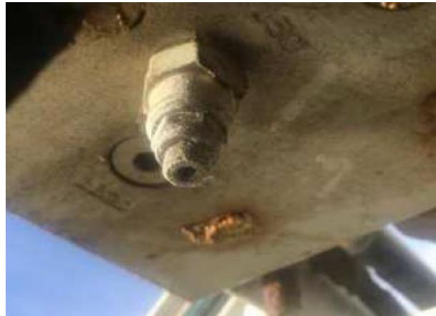
Second valve set incorrectly
