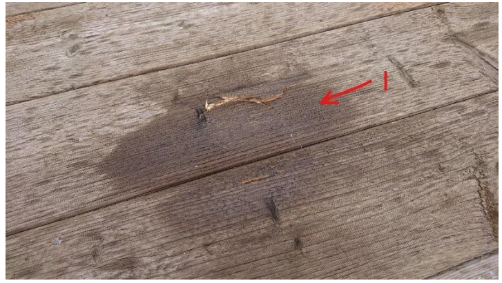
Dents in the wooden deck
