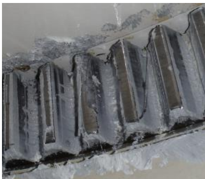
Pinion gear damage
