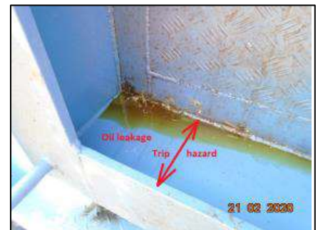
Hydraulic oil leak
