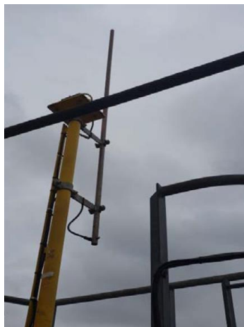
Mast and lightning conductor
