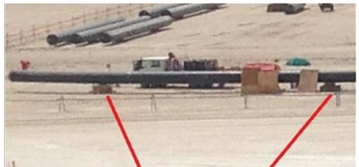
Position of pipe before falling from the two supports pictured (of eight total)
