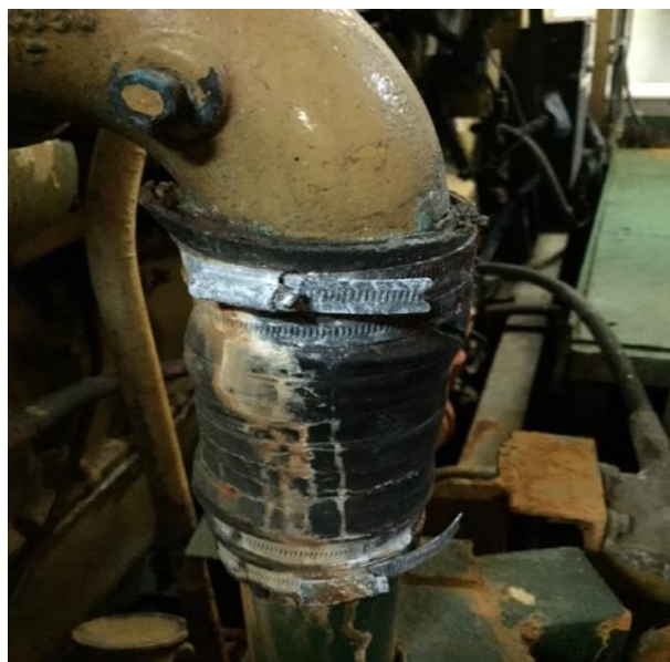
Hose clamp condition - in use on suction side of sea water cooling pump, found on the day of investigation, on the same engine where the failure occurred
