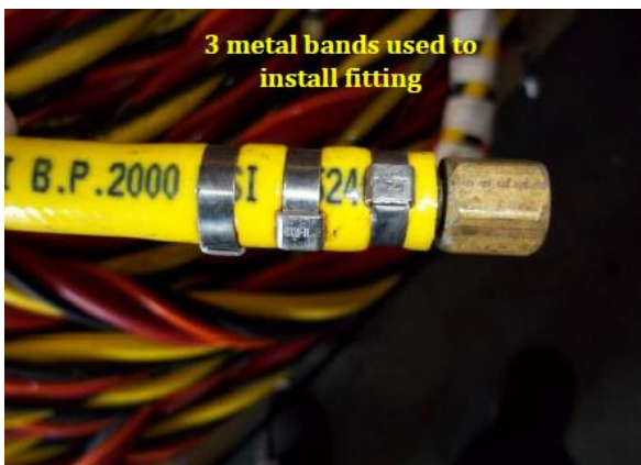
Fittings on 3/8" Gas Hoses (HDA0106) were installed with three metal bands;
