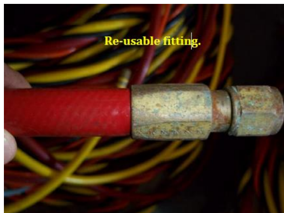
Fitting installed on the 1/2" Hot Water Hose (HDA1108) were re-usable fittings.
