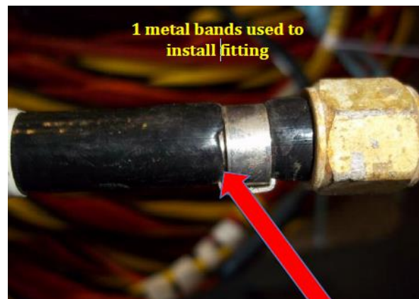
Fittings on the 1/4" Pneumo Hose (HDA0104) were installed with a single metal band; Red arrow indicating cut jacket, exposing braid
