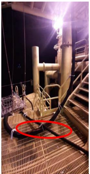
Position of temporary hoses at incident scene
