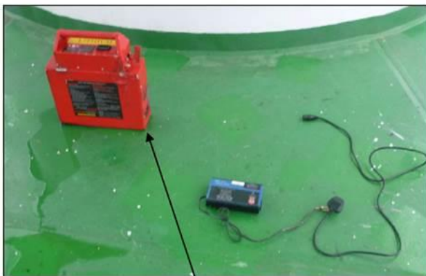
Failed unit and charging cable
