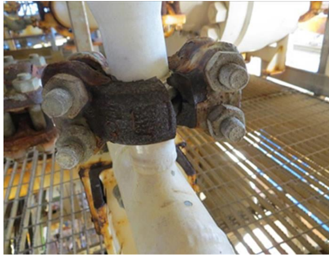
Cracking caused by poor heat treatment during manufacturing process.
