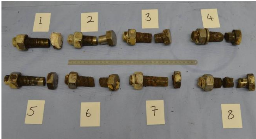
The condition of the severed bolts.
