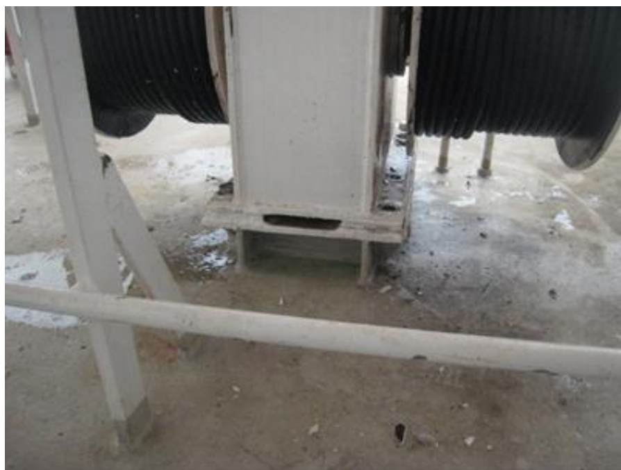
Winch foundation plate assembly (with some failed bolts removed).
