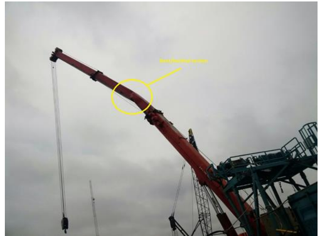
Showing point at which crane boom buckled (marked)
