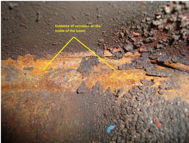
Showing close-up of corrosion
