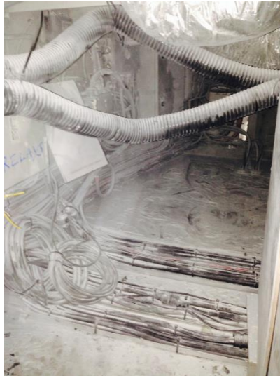
Figure: damage caused by dry powder extinguishers
