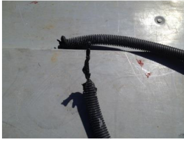
Figure: main control cable conduit burned through
