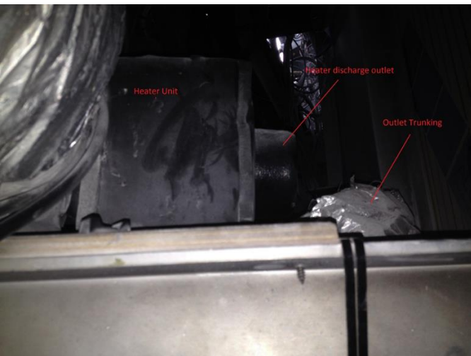
Figure: main discharge trunking from the heater system was seen to have become disconnected from the heater
