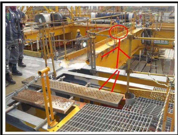
Showing from where and how injured person fell
