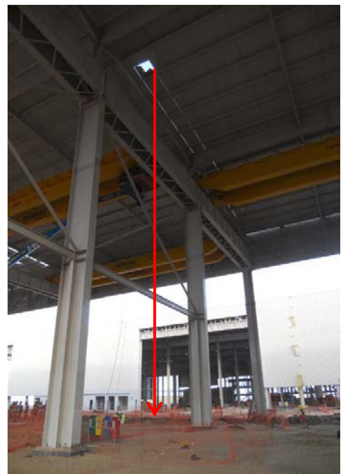
Showing the hole through which person fell and the distance to ground
