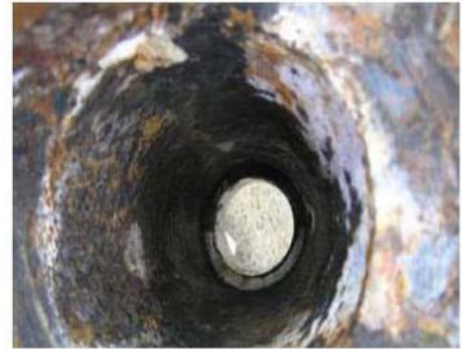
The surface of the inner cone was corroded and rough, although loose rust was removed
