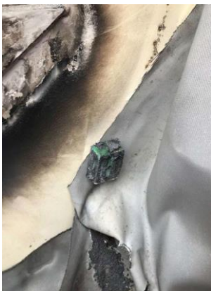
A magnet used to secure fire protection
