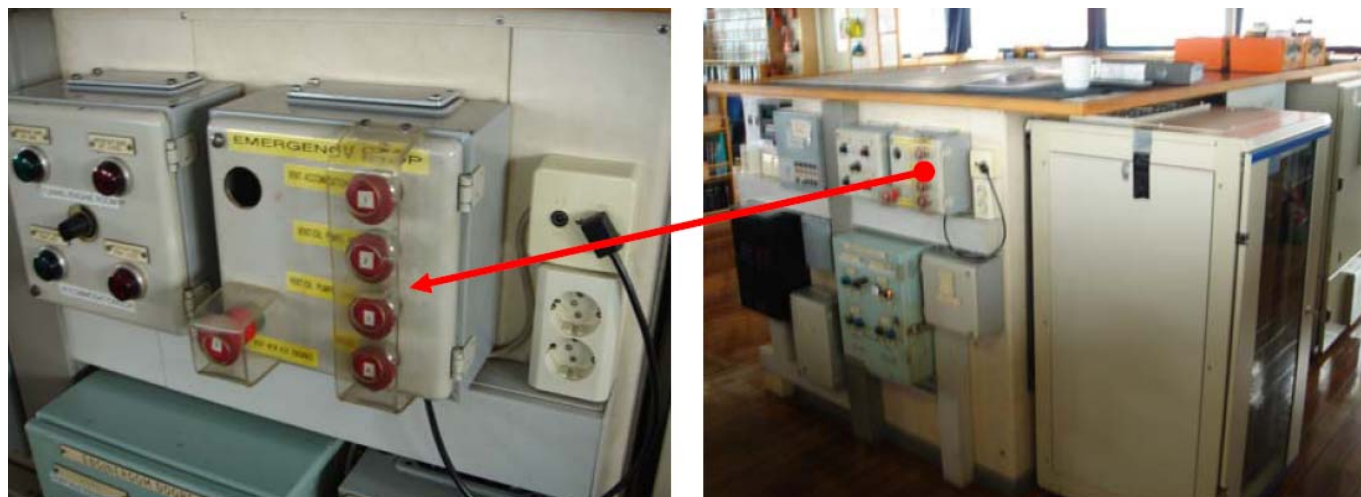
Emergency power switches
