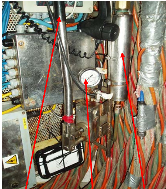
Pump handle Gauge Hydraulic reservoir
