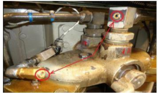
Failed connection as found by duty engineer
