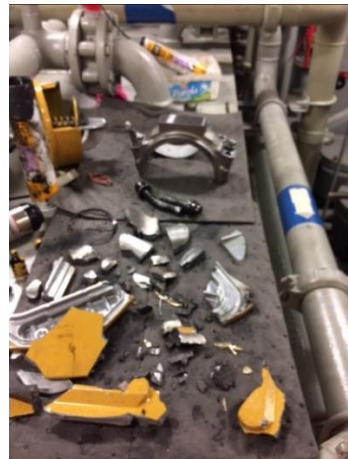
Debris found spread around the engine room
