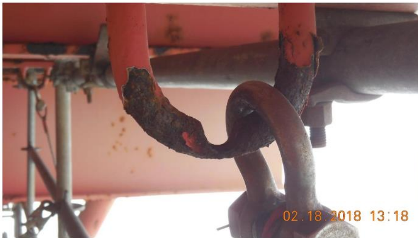
BSEE inspector's photograph of swing rope in place on a Gulf of Mexico facility
