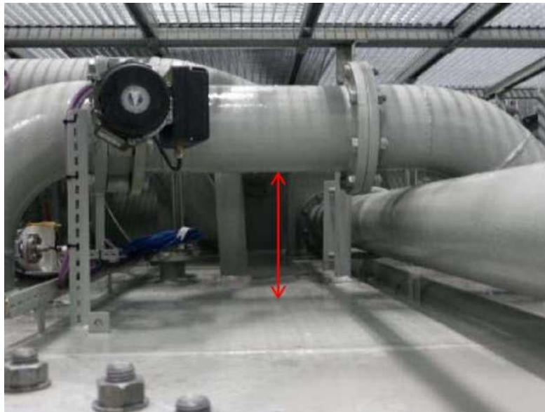
Figure: Showing area against which crewman was pushed by flow of water. NB height from deck to the pipe is approximately 0.35m (red arrow)
