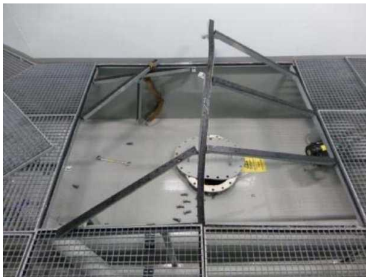
Figure: Showing damaged grating and manhole from starboard side.
