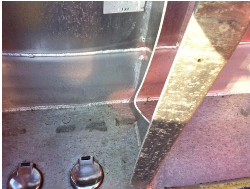
Figure: Showing buckled frame and bent plate, as a result of collision between wind farm service vessel and turbine foundation
