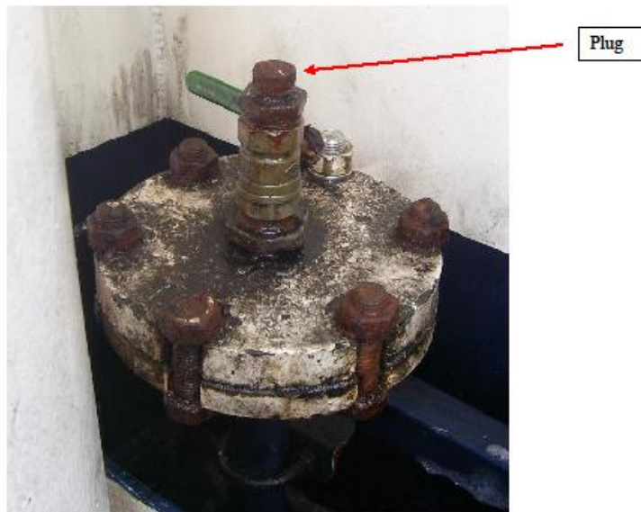
Starboard Waste Oil Connection
