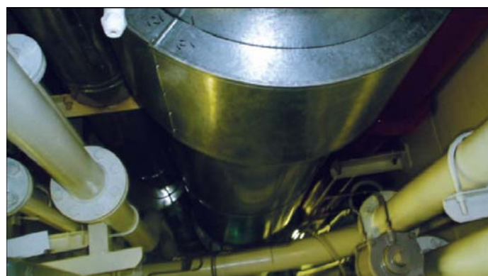
Picture 2 – Exhaust pipe
