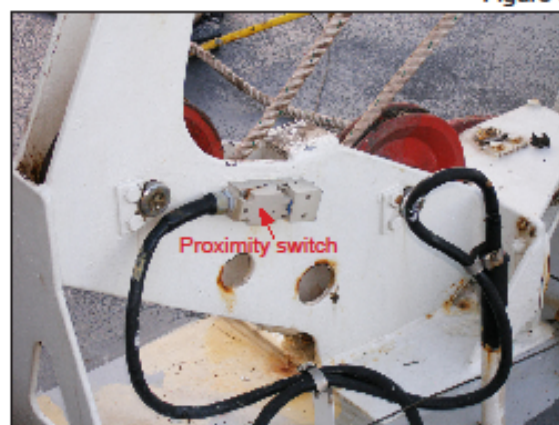
Proximity switch on davit
