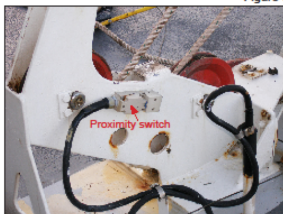
Proximity switch on davit
