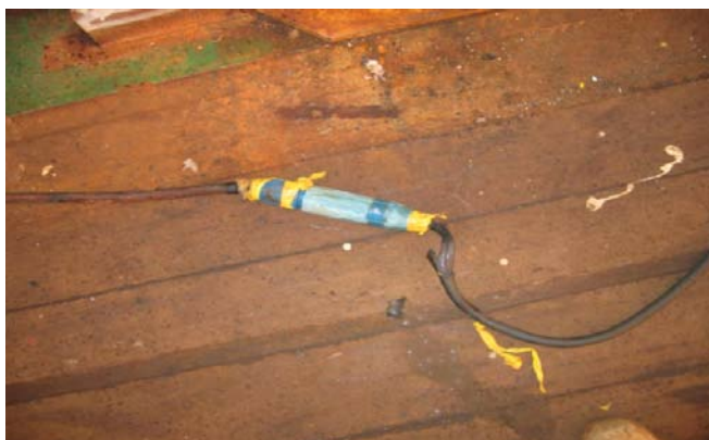
Figure 3 – Welding cable found to be smouldering
