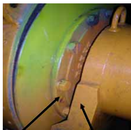
Rotating ring of bolts Stationary winch base Figure 2 – Detail of gap between winch drum cheek plate and the winch base
