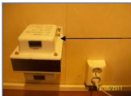
Transformer 220v – 110v purchased in USA for running machine.
