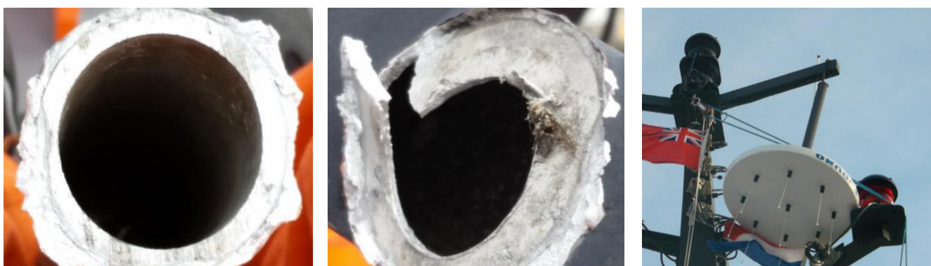
Figures: photographs of mast damage following the second incident
