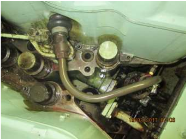
Top view of the failed pipe in place
