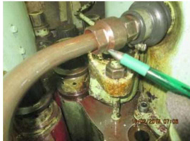
Location of failure at the fuel pipe coupling
