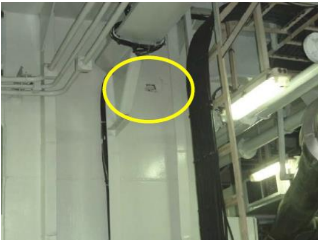
Figure: Damage to engine room wall (other side of moonpool) following stopper bar broken
