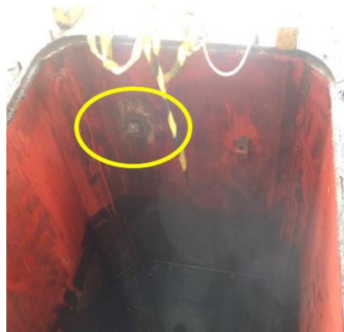
Figure: Damage to side of moonpool after stopper bar was broken
