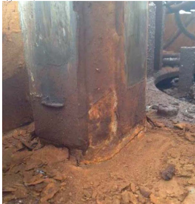
Figure: (Above) showing cracked welds
