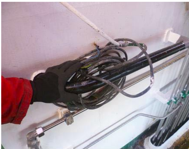
Figure: showing electrical cable and bare live wires
