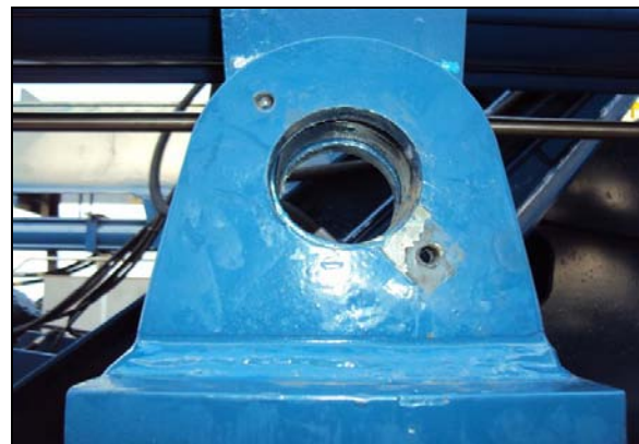
Lift post pin missing
