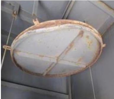
Poor sealing of fire damper
