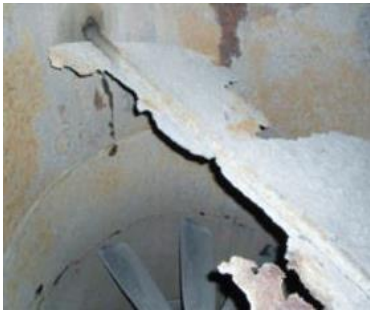
Corroded engine room fire damper
