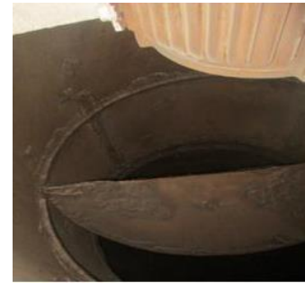
Broken flap on engine room fire damper
