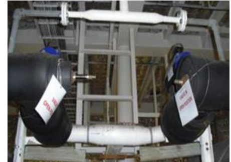
Low pressure valves for CO 2 system kept closed
