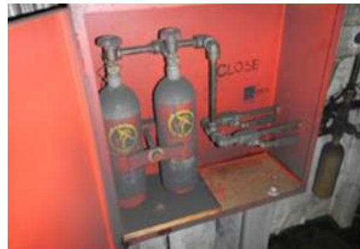
Faulty CO 2 actuation valves
