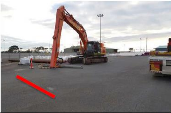
Image 1: Showing Excavator (left) and location of trailer (right). Red line showing location where line pipe was dropped. Uncoated line pipe can be seen to left of excavator
