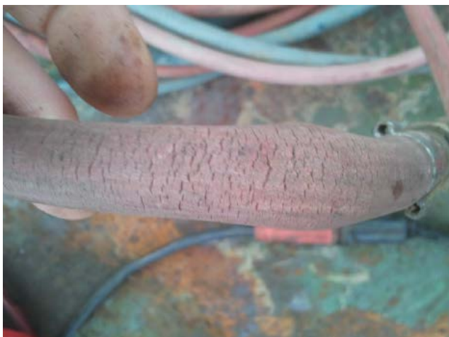
Work-hardened and perished hose
