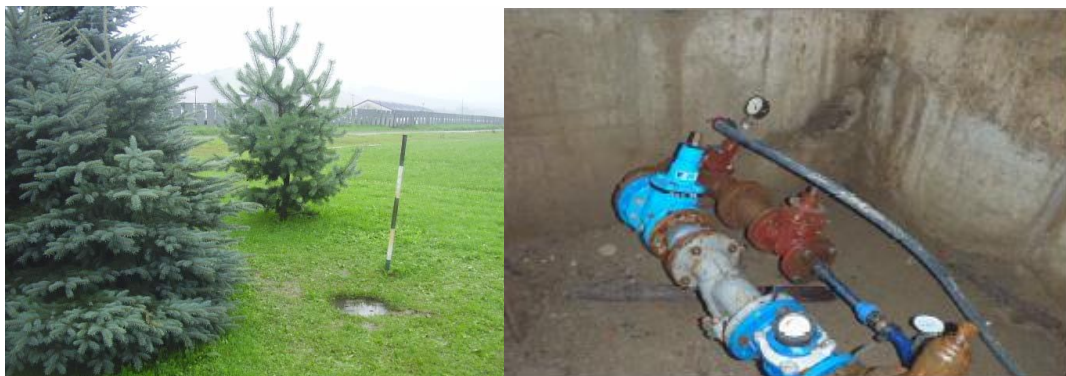
Entrance to confined space and view into confined space showing water meter
