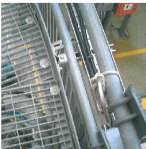
Showing spade secured to handrail and view to deck below
