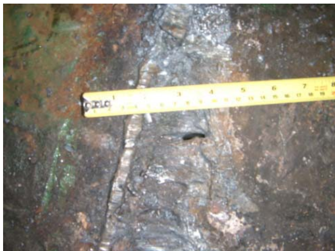
Hole burnt in deck
