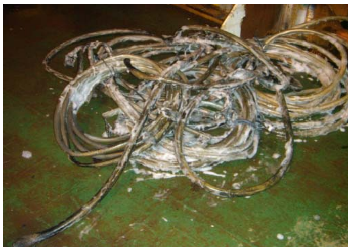
Damaged plastic hose in space underneath
